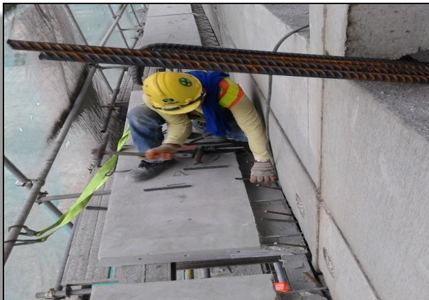
AC Ledge Installation, Amaia, Pasig City
